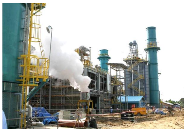
Steam blow commissioning at the Sengkang Power Plant (Block 2), 180 MW capacity after expansion
