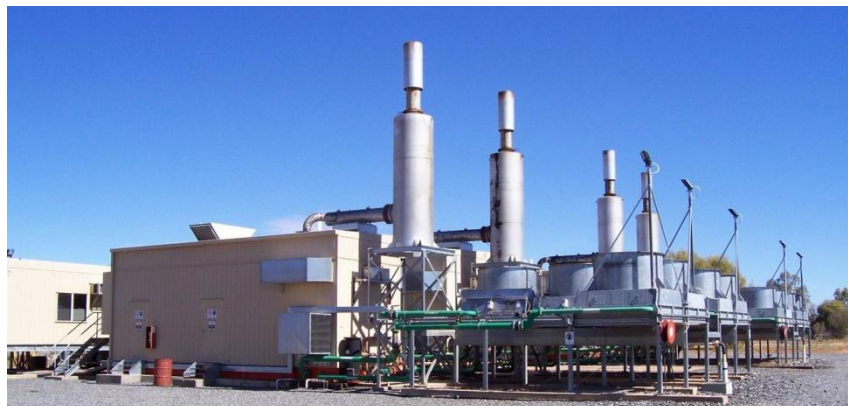
Alice Springs Power Plant, Australia
