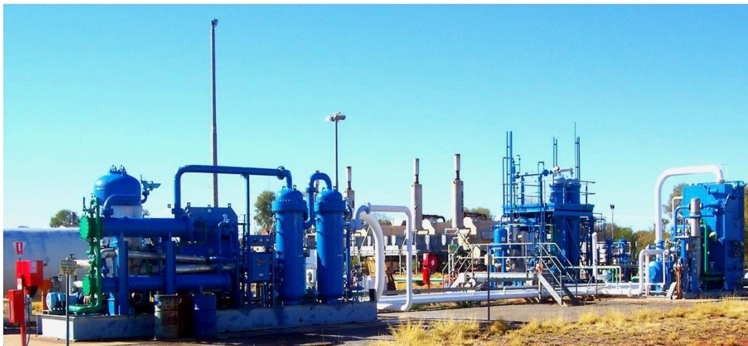
PPU and cold box at Alice Springs LNG Facility, Australia
