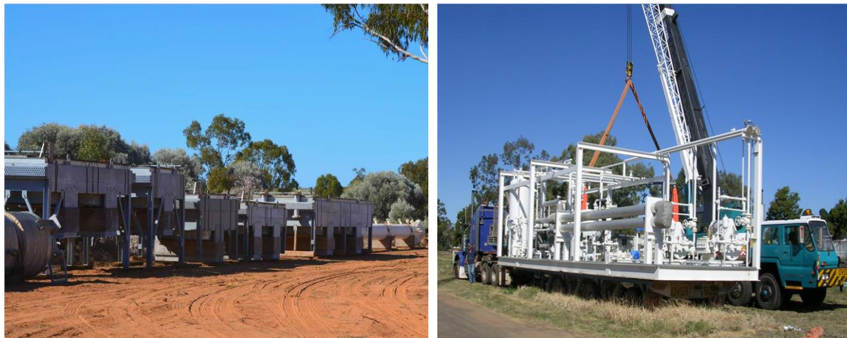
Equipment at the Gilmore LNG site
