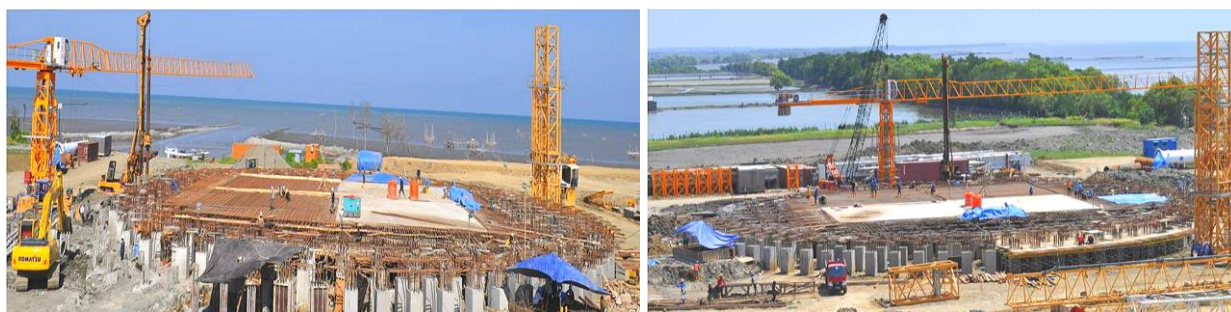
Construction of bore-piles and pile heads with base slab works in progress
